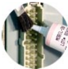
k. Secondary Disconnect Receptacle
