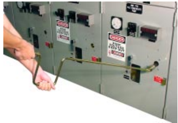
Figure 14. Racking the PowlVac-ND® Circuit Breaker
