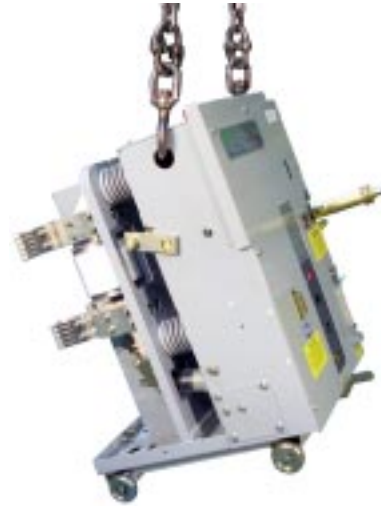
Figure 10. Circuit Breaker and Crane
