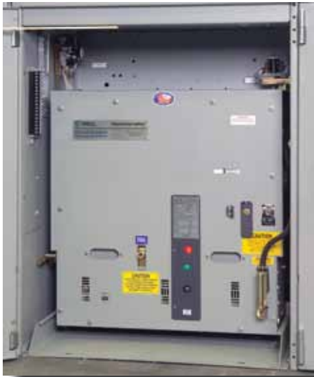
Figure 13 Circuit Breaker in Test Position
