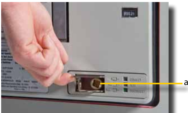
Figure 4 Close-Up Racking Shaft Position
