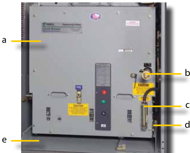
a. Circuit Breaker in Compartment b. Racking Mechanism c. Secondary Disconnect d. Anti-Rollout Latch e. Compartment Floor
