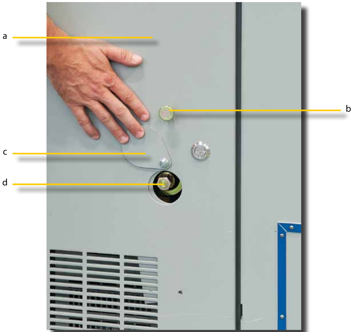
Figure 5 Switchgear Compartment Door
