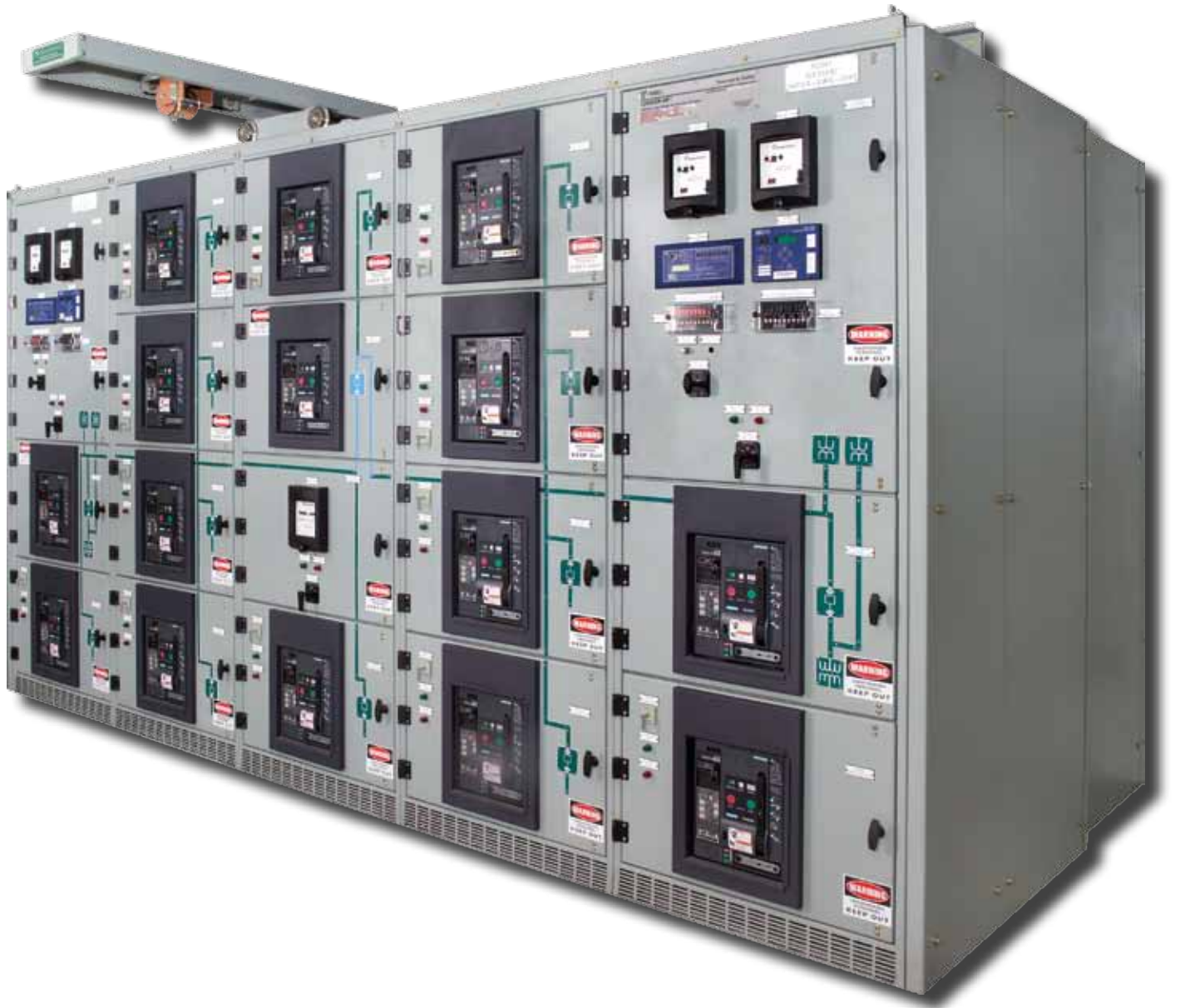
Figure 1 Powell Low Voltage, Arc Resistant Switchgear
